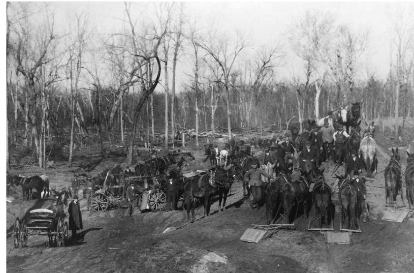
[Fig. 41] 1888 Brevoort Levee construction with slip-scrapers with Brevoort far left (in library)
